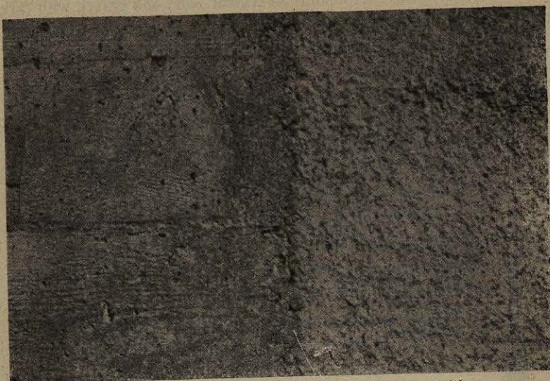
Surface left by forms is shown on left and picked surface on right. FIG. 105.—Surface of "Picked" Concrete. (See p. 289.)
