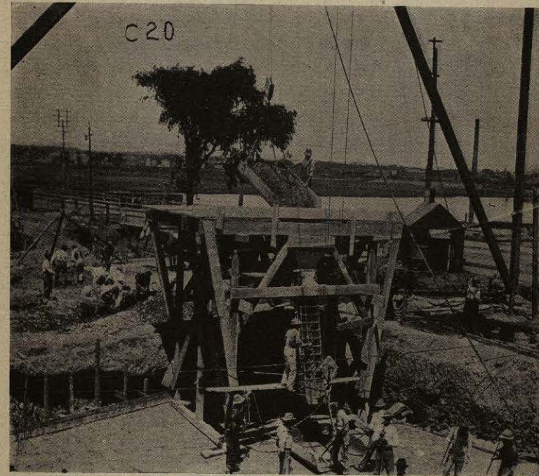
FIG. 93.—Portable Mixing Plant. (See p. 271.)
