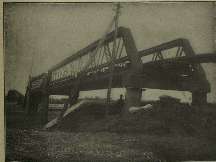
FIG. 242. — Damage to a railroad bridge by the Japanese earthquake of 1891. Note how the earth was shaken from beneath the track where it leaves the bridge.
